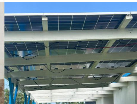
Solar panels adjacent to main building
